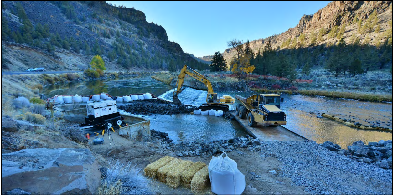
Figure 4-4. A trackhoe with a bucket and hydraulic thumb loads a dump truck with broken concrete for hauling off-site during a dam removal project.
