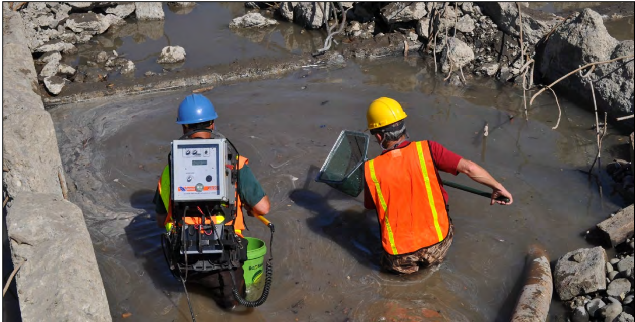
Figure 4-2. Two-person crew uses a backpack electroshocker and dip nets to salvage fish from work area during a concrete dam removal project.
