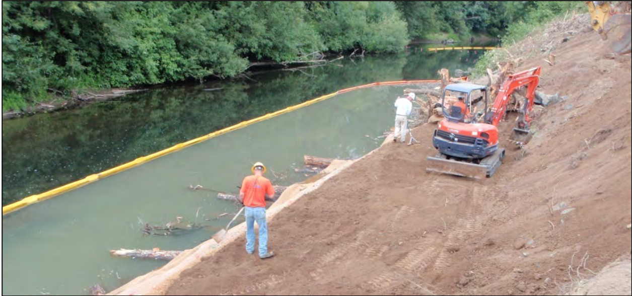
Figure 4-5. An example of a floating silt curtain isolating an active work area from clean water flowing by the project site. Turbid water is contained within the work area by the silt curtain.
