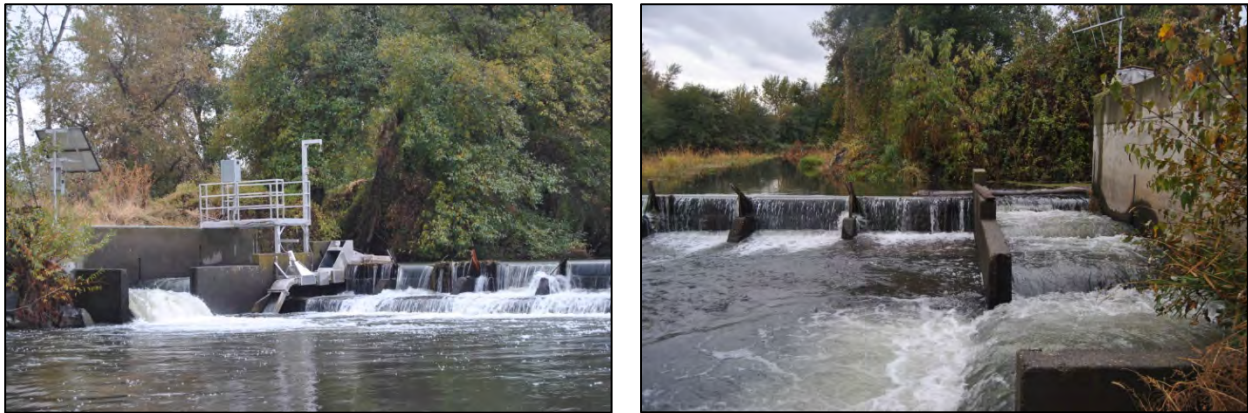
Figure 2-1. Upstream views of existing fish ladders on each side of existing Dillon Dam.
