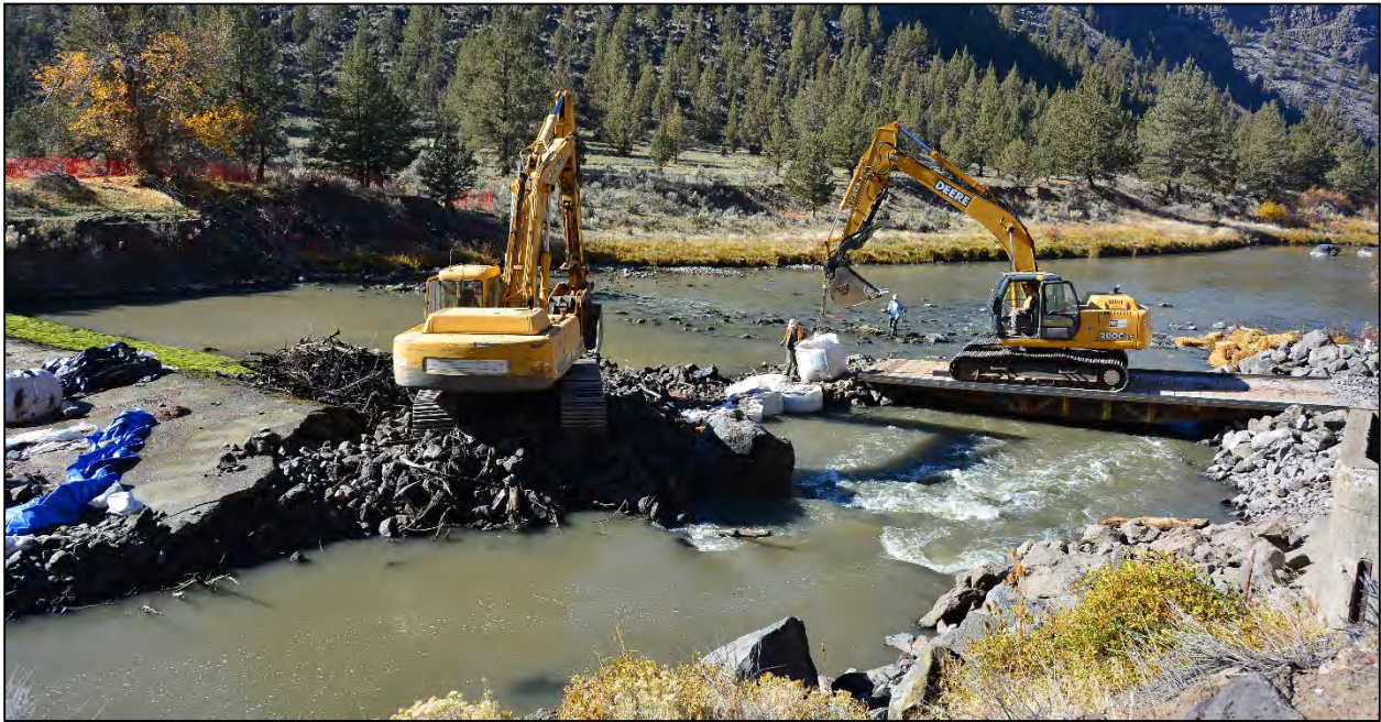
Figure 4-6. An example of a temporary bridge installed over an active channel to access the opposite side of the river for dam removal and restoration work.
